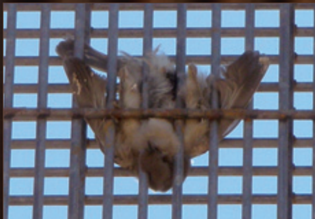
This unfortunate bird perished after becoming trapped in the steel barrier running through Organ Pipe Cactus National Monument in Arizona.
